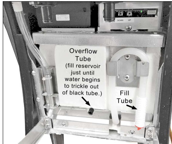
Figure 4-2 - Ice Bank Fill & Overflow Tubes
